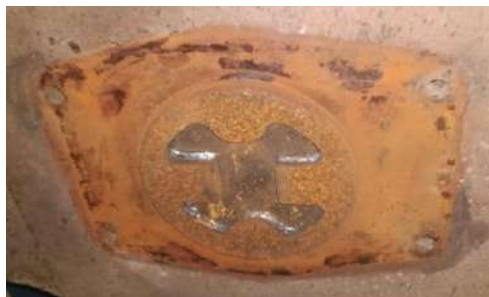
Figure 14 Spherical CP top mounting location examination-Surface shall be examined for any crack etc. and attended as per relevant repair procedure of body bolster for the respective wagon
