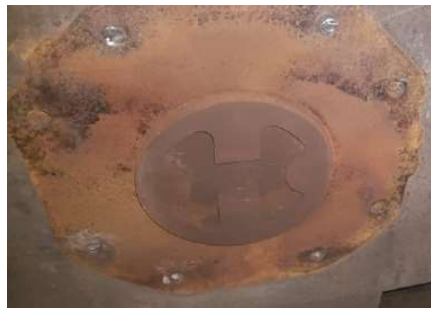
Figure 30 Flat CP top mounting location examination- Surface shall be examined for any crack etc. and attended as per relevant repair procedure of body bolster of the respective wagon
