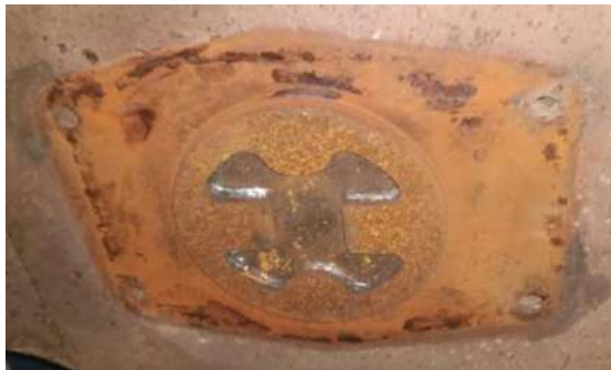
Figure 24 Spherical CP top mounting location examination- Surface shall be examined for any crack etc. and attended as per relevant repair procedure of body bolster for the respective wagon
