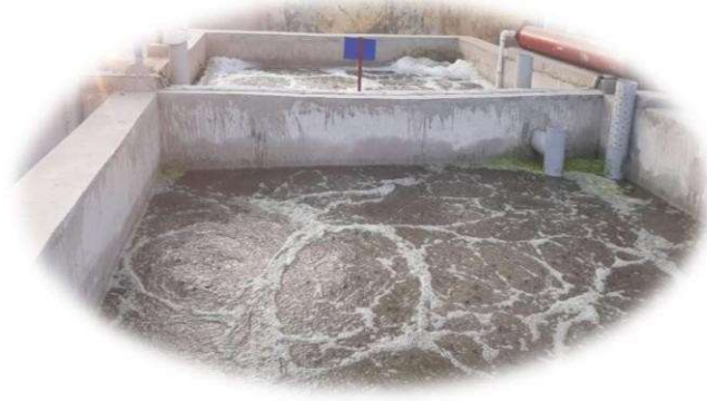
WATER RECYCLING PLANT
