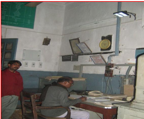
LED lighting through solar at Wazirganj
