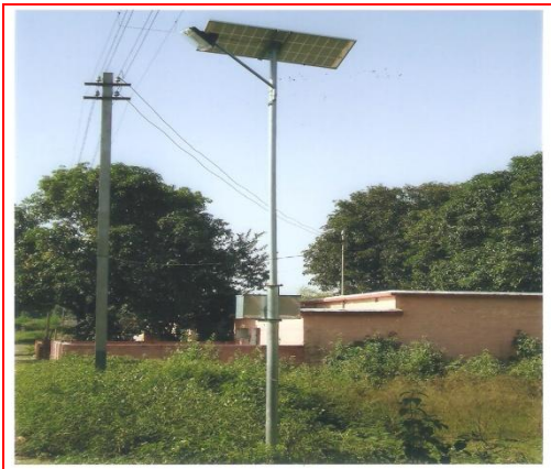
Street light through solar at MDJ
