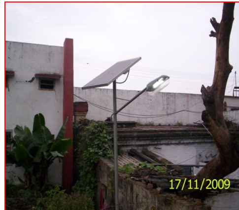
Street light through solar at Bapudham
