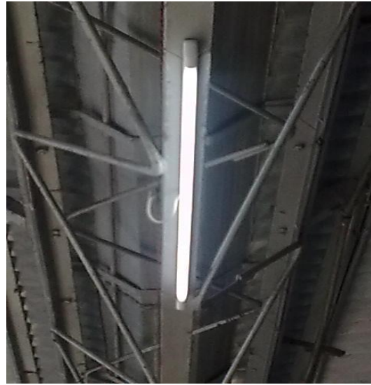
T5 Tube light at SPJ Station
