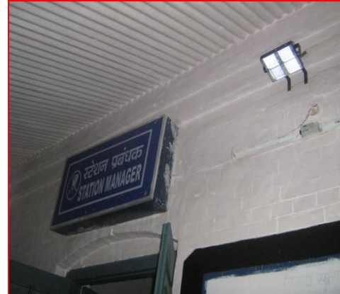
LED lighting through solar at Wazirganj
