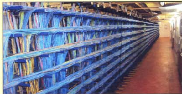
Fig-4: Complex and Intricate Wiring of RRI LED Signals
