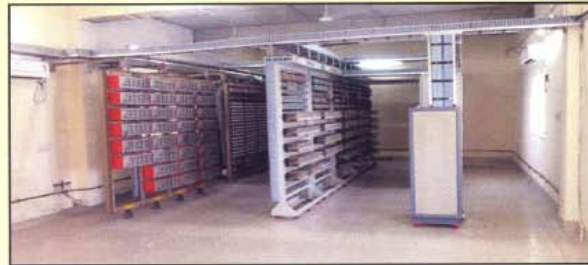
Fig-2: EI Relay Room
