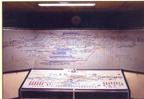
Fig-3: RRI Operations Panel and RRI Indication Panel
