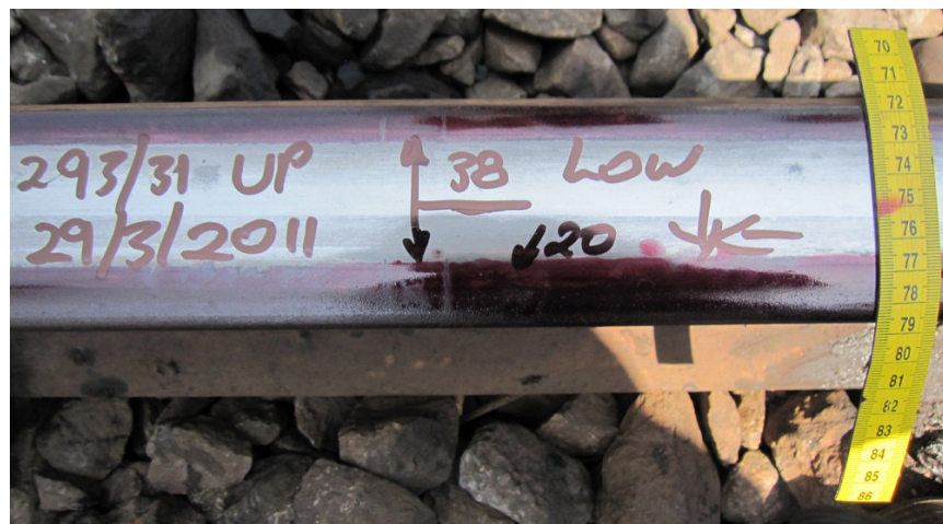
Fig. 32: Photograph Showing Contact Band Details after Grinding
