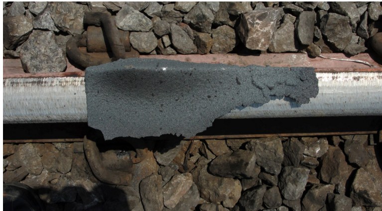
Fig. 12: Accumulated Rail Dust Lump
