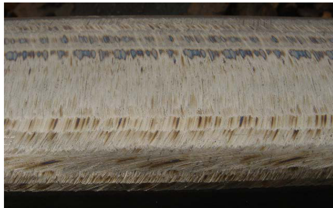
Fig. 37: Poor Surface Finish
