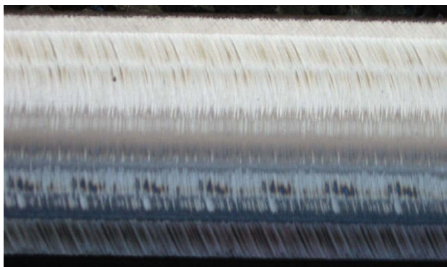
Fig. 35: Skipped Grinding & Blueing of Rail
